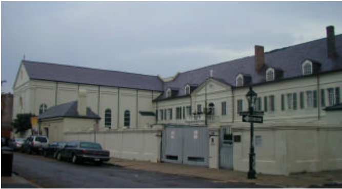
The Early 18th Century Ursuline Convent in New Orleans. The church roof was lifted and dropped by Katrina.
